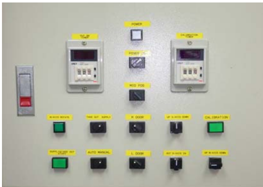
Fig. 14. The control panel.
